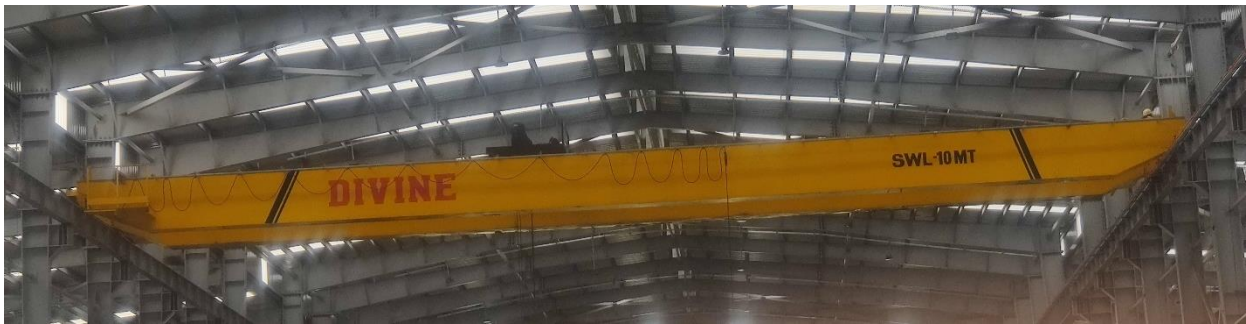
Fig 2. 10 Electric Hoist Travelling Crane
