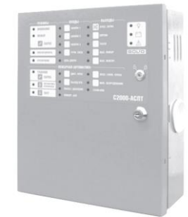
FIRE ALARM SYSTEM
